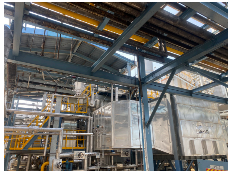
New boiler facility expansion
