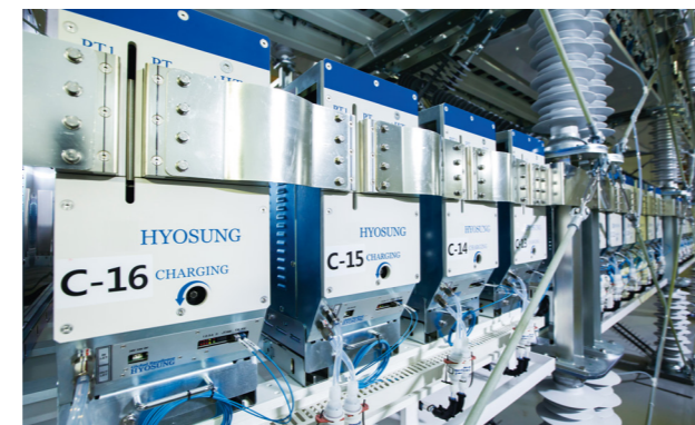
Static Synchronous Compensation (STATCOM) by Hyosung Heavy Industries
