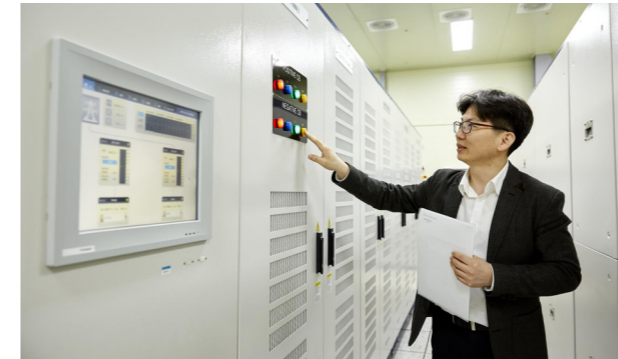
Energy Storage System (ESS) by Hyosung Heavy Industries
